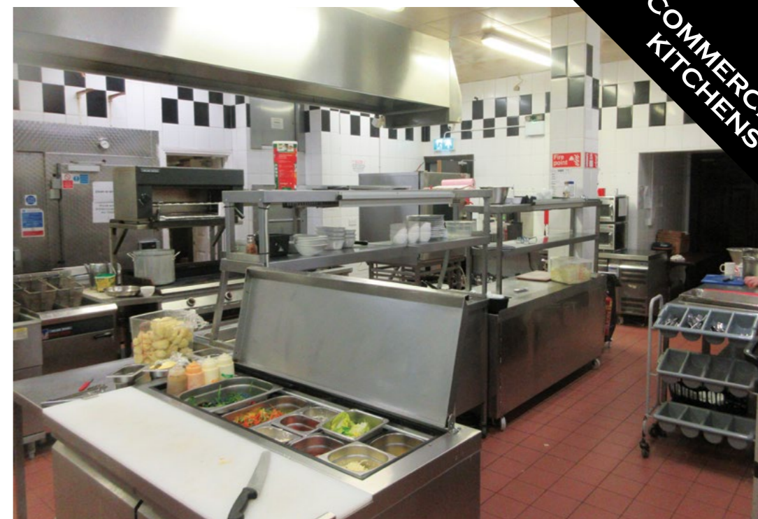
One of two commercial kitchens at the Bay View Hotel in County Donegal, this large room provides plenty of space for staff to work in without hindering each other in any way, as should always be the case in any busy commercial kitchen.
